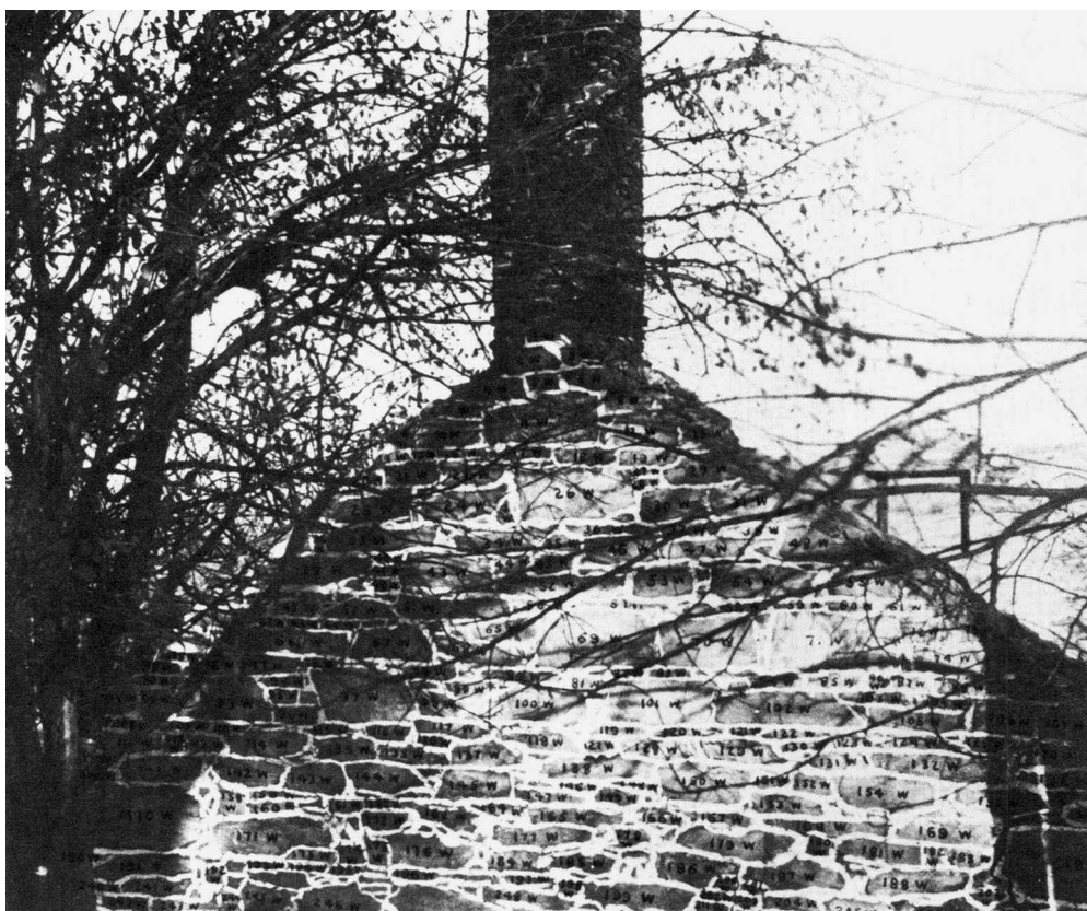
fig. 22. Every stone of a nineteenth-century cottage in South Burlington is numbered before the cottage is dismantled and reassembled on the museum grounds, 1950 [Shelburne Museum]
